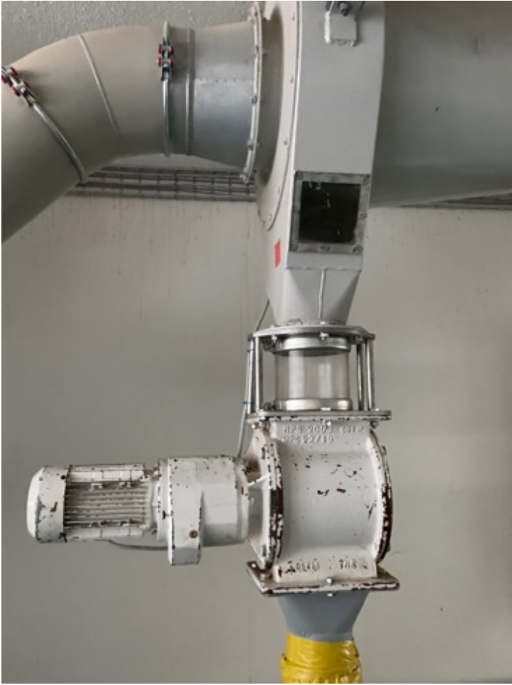
Cyclone and rotary gate
