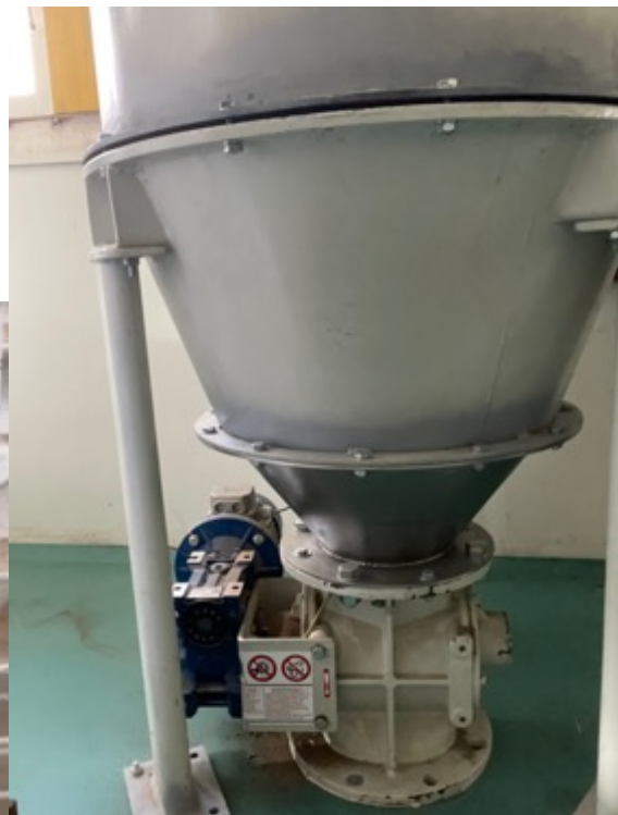
Drive of the rotary valve at the outlet of the filtered fraction
