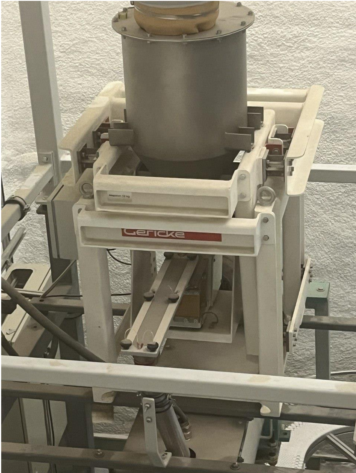
Gericke loss-in-weight-feeder mounted in the automated feed dosing station
